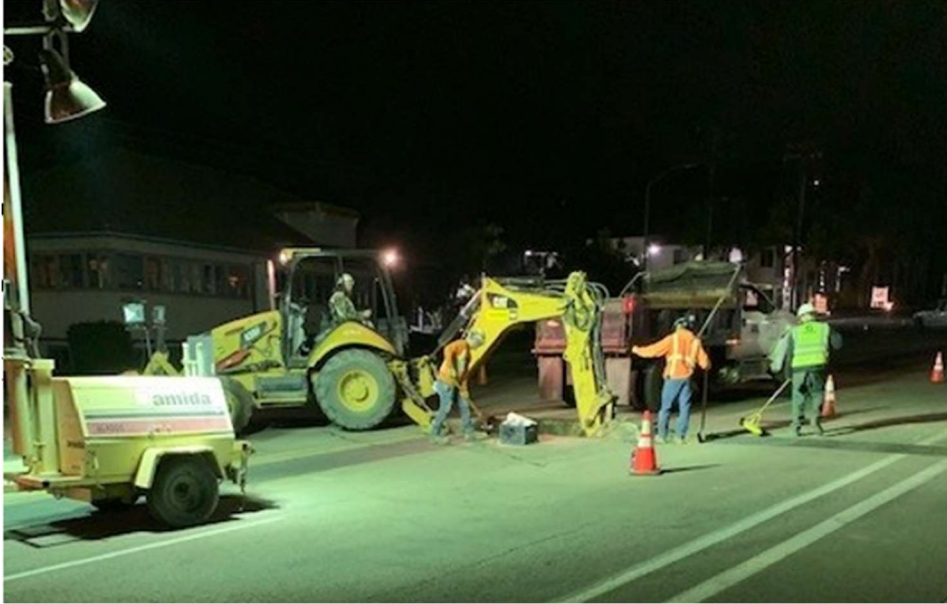
Night crew working to install new potable water pipeline along Manchester Avenue
