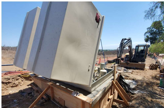
Newly installed pressure reducing stations at Lone Jack location
