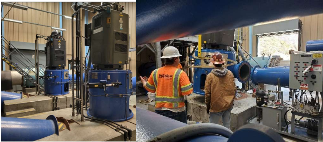
Refurbished turbines being reinstalled at the District's David C. McCollom Water Treatment Plant
